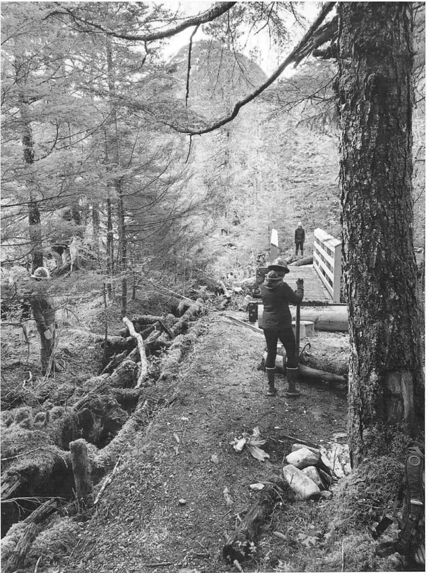
Trail Mix crew members Justine Webb, Sarah Wallace and Allison Mickleson move bridge approach timbers into place. (Courtesy photo / Ryan O'Shaughnessy)
